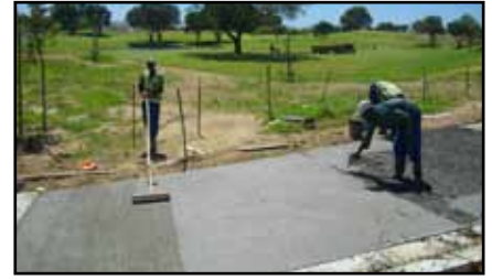
The cart paths are brushed with a stiff broom while they are still wet to slightly roughen the surface and provide texture
