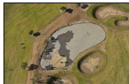
Aerial photograph showing the installation of the gravel blanket to the 3rd green
